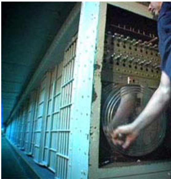
Added to this excerpts presentation, from the CorrectionHistory.Org website, the above image shows "the wheel" being operated to open or close cell doors.
