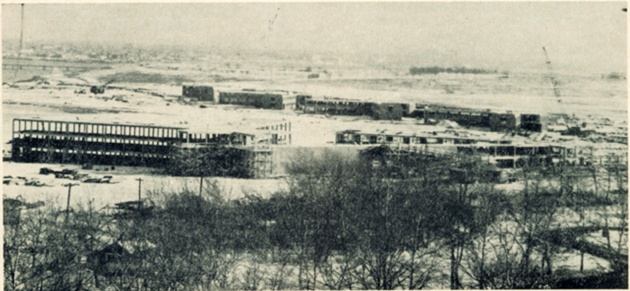
IT IS BECOMING A REALITY ... The New York City Correctional Institution for Women, to be built at a total estimated cost of $23,652,000, is moving towards its completion date in 1969. Photo taken December 1967.
